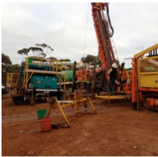
SRU in Kalgoorlie, Western Australia
