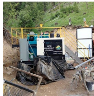
SRU in Montana, USA
