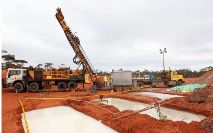
Traditional drilling fluid sumps
