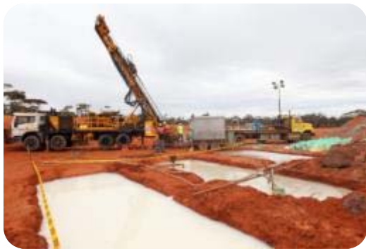
Traditional drilling fluid sumps
