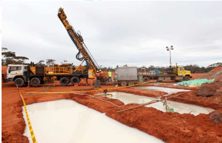
Traditional drilling fluid sumps
